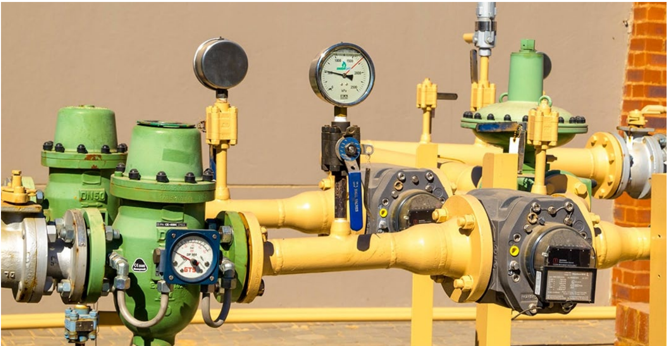
Pressure control Valves and Shut-off Valves
